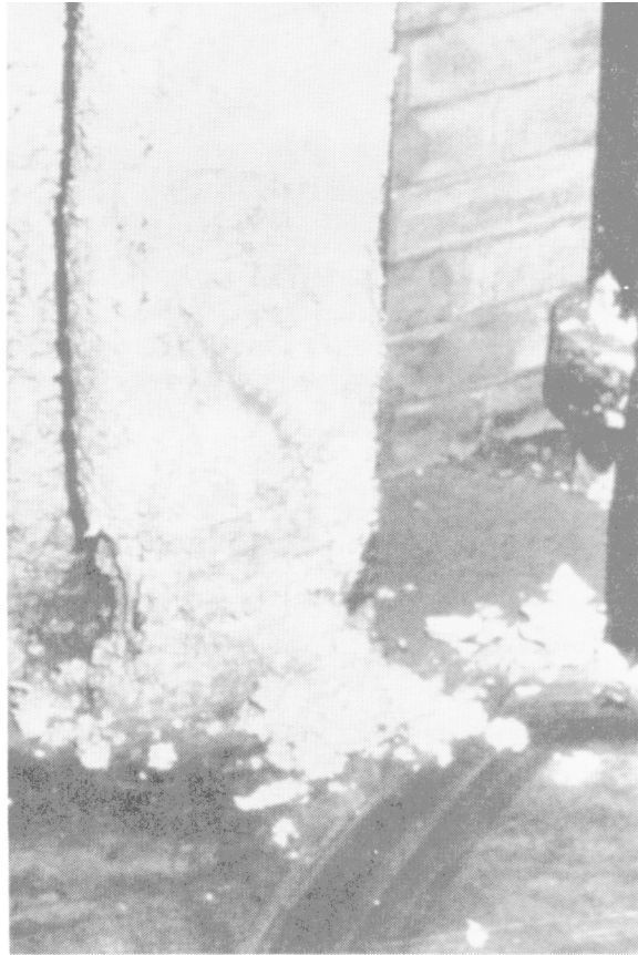
ACM which is in poor physical condition. Under a proper operations and maintenance program, corrective action would normally prevent deterioration of the insulation.
